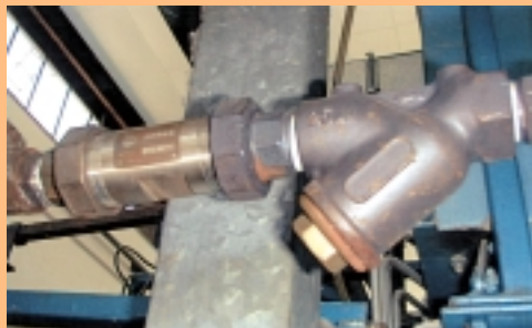
A GEM trap installed at Withington Hospital laundry
